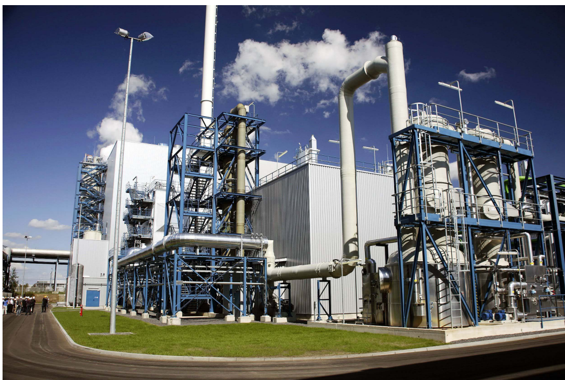
CCS pilot installation in Jaenschwalde, Germany
