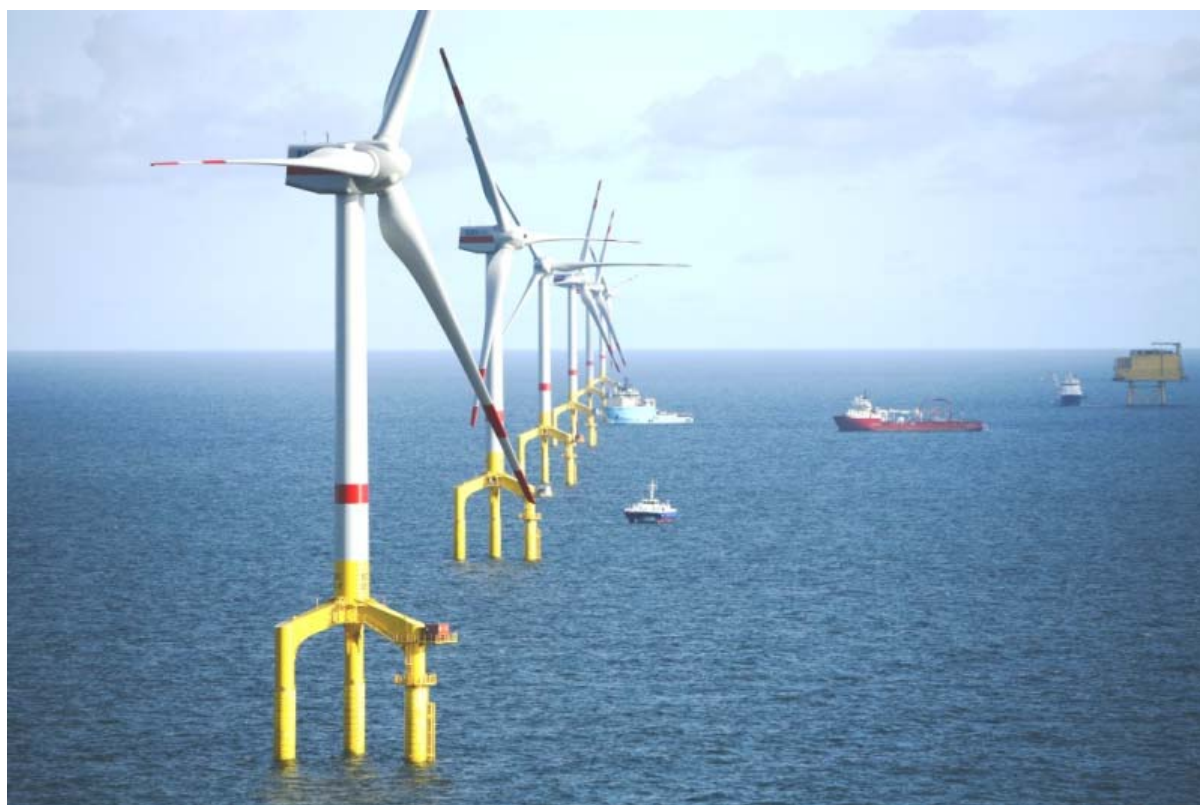
Multi-MW turbines and offshore foundation structures, co-financed by the EEPR, installed at the Bard I site in the German North Sea
